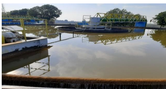
Fig.2: A view of sedimentation tank in operation
